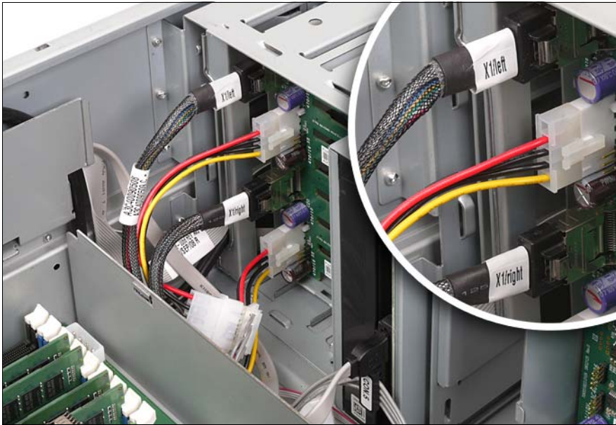
Figure 47: Cabling 2.5-inch HDD extension box
